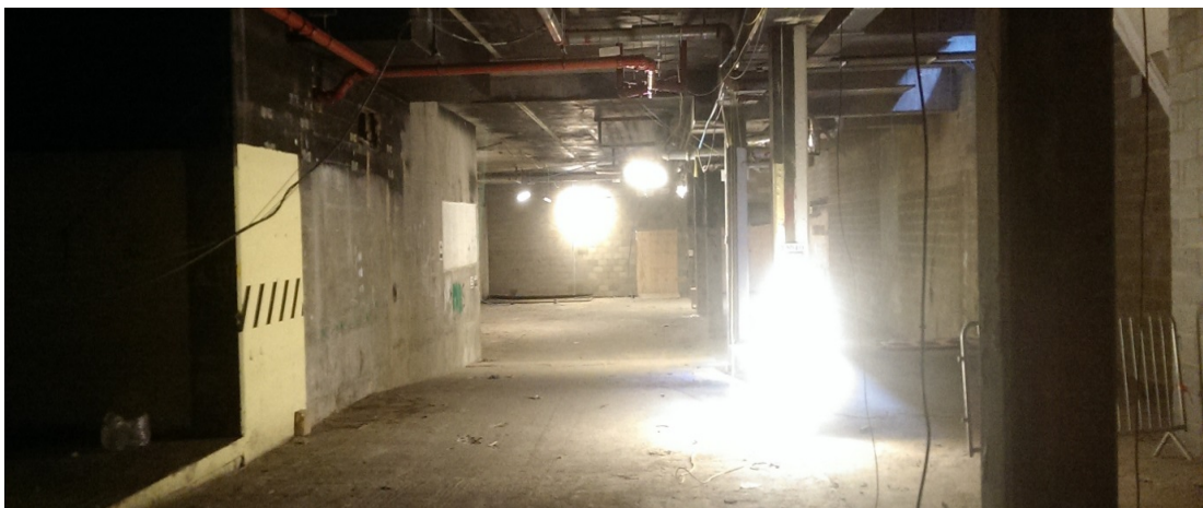
Figure 2 (a): Basement level 3 (historically used for plant equipment for the entire building)
